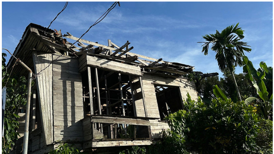
Figure 1. Public infrastructures and houses damaged by Super Typhoon Rai, also known as Odette
